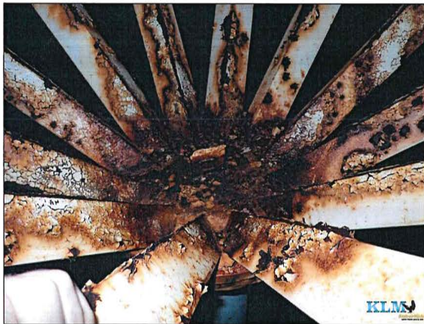
Photo No. 4 Condition of top of center support column
