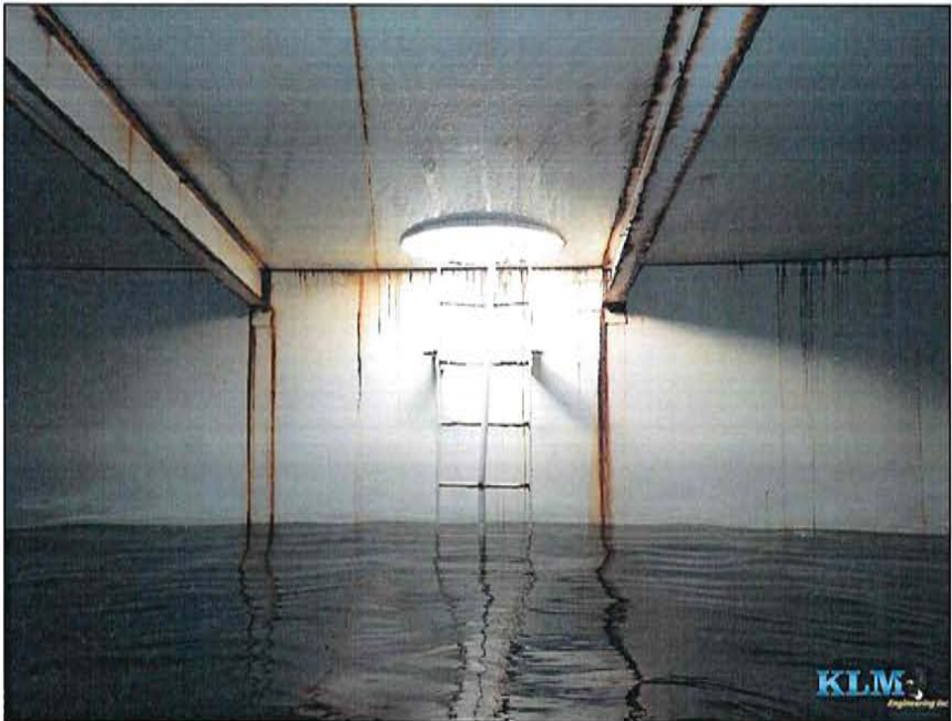
Photo No. 12 Interior wet ladder
