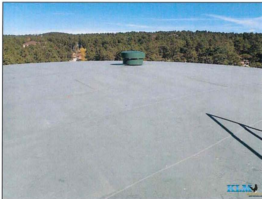
Photo No. 14 Condition of roof coating
