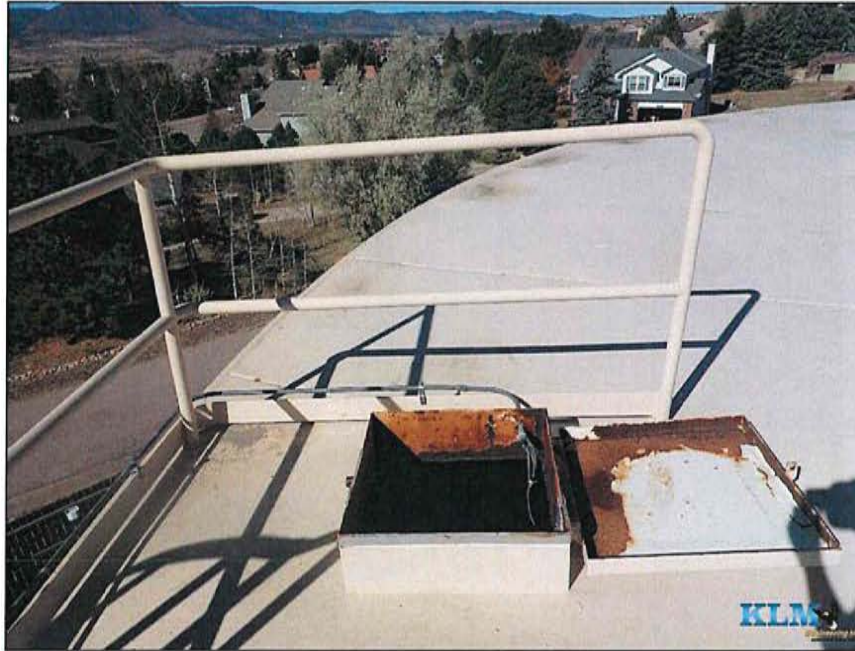
Photo No. 17 Condition handrail and wet access manway
