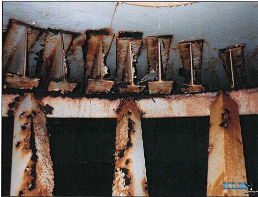
Photo No. 5 Condition of roof rafters and connection ring
