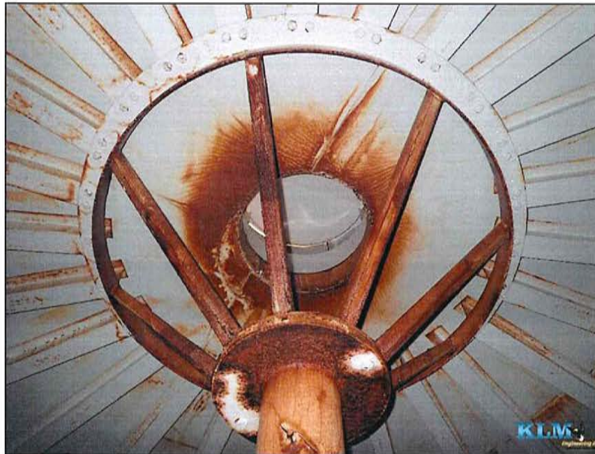
Photo No. 3 Condition of dollar plate and top of center support column
