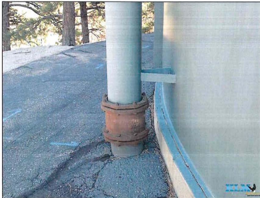
Photo No. 24 Overflow pipe
