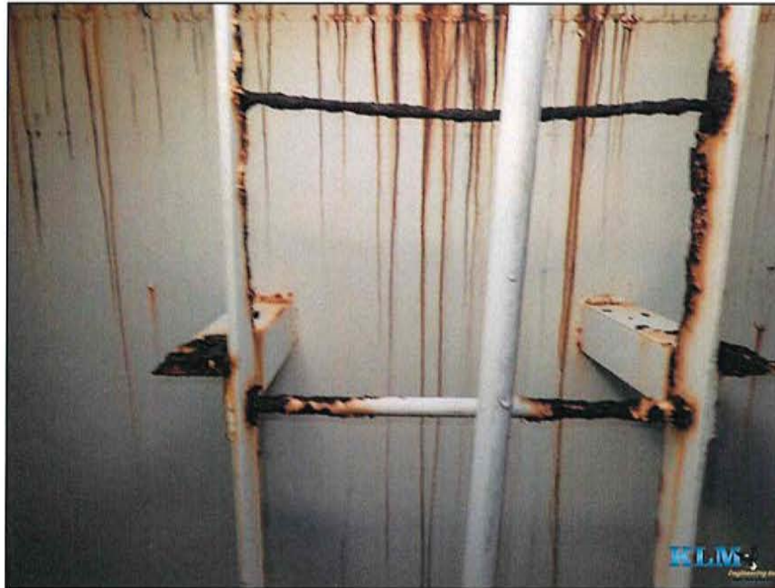
Photo No. 13 Severe metal loss on ladder rungs
