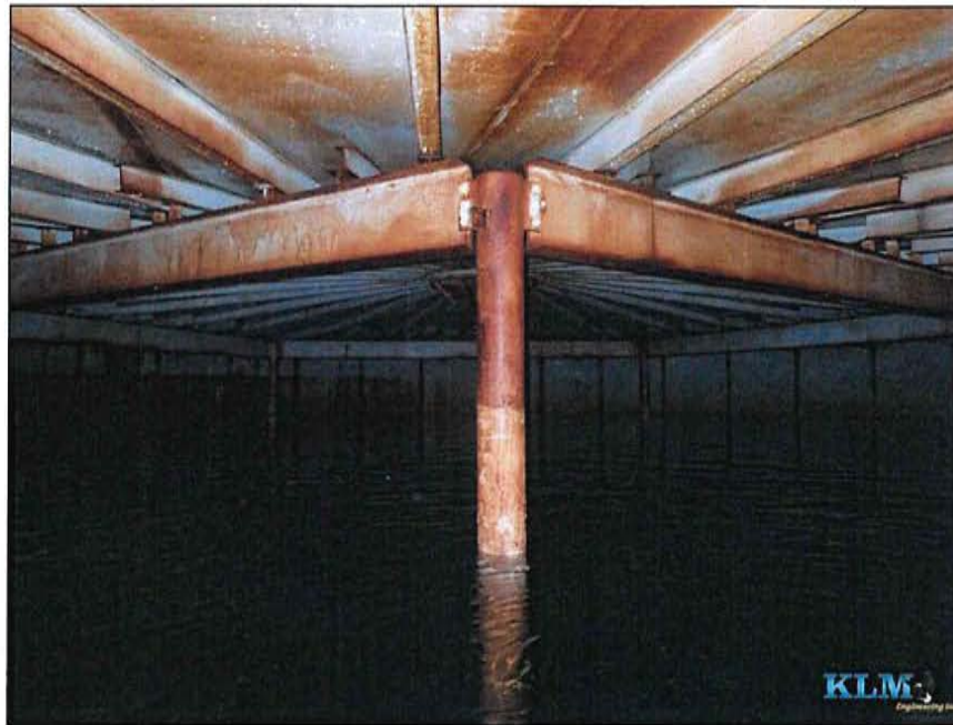
Photo No. 5 Condition of roof plates, roof rafters, and support column
