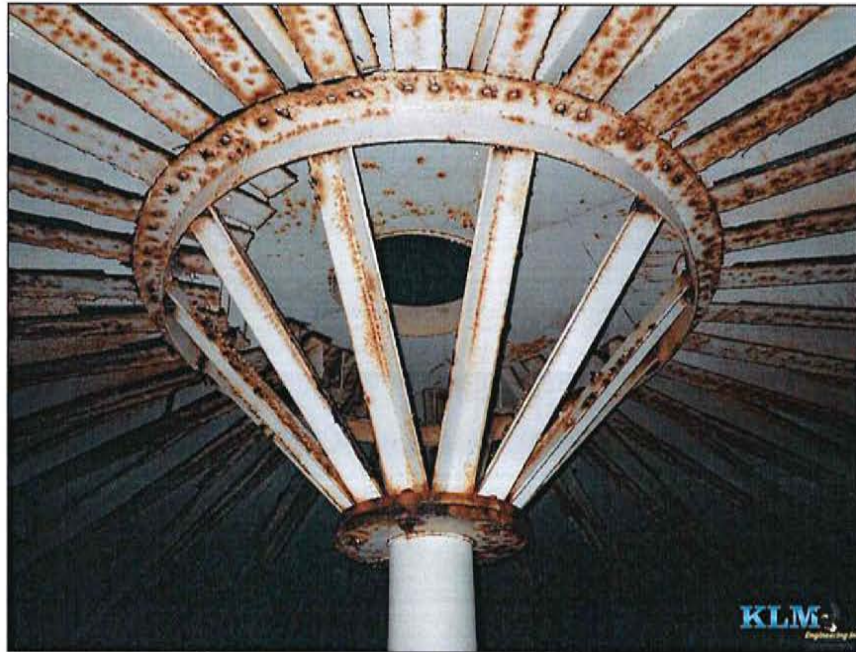
Photo No. 3 Condition of dollar plate and top of center support column
