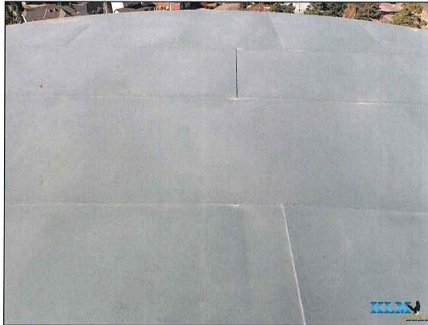
Photo No. 17 Condition of roof coating
