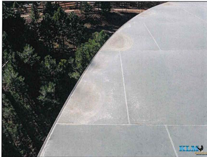
Photo No. 13 Condition of roof coating
