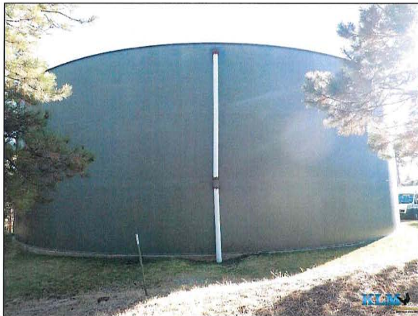
Photo No. 18 Condition of shell coating Overflow pipe visible
