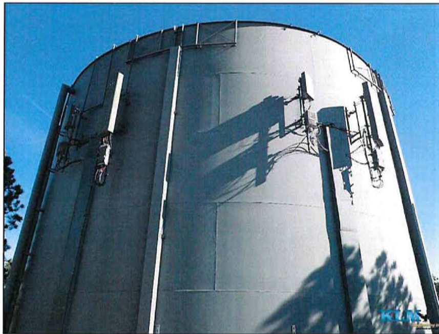
Photo No. 22 Condition of shell coating
