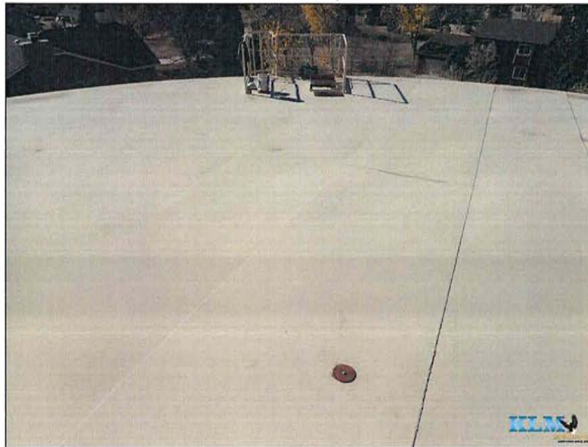
Photo No. 15 Condition of roof coating
