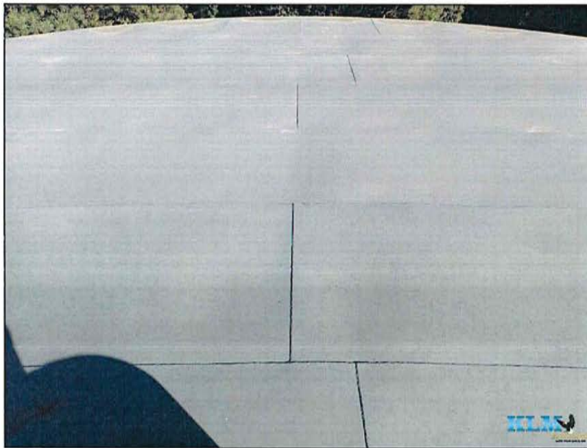
Photo No. 12 Condition of roof coating
